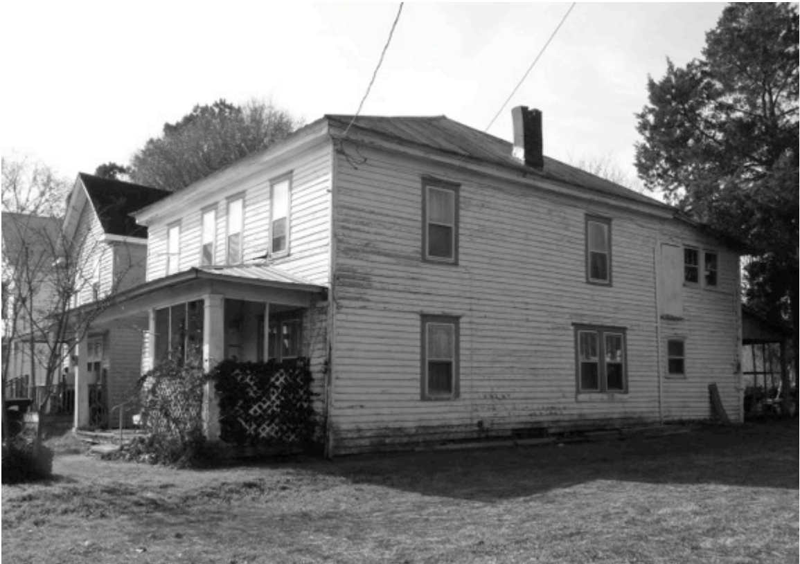
Fig. 8: A water line, approximately one meter above the foundation, on a historic residence in Shepard Street Historic District indicates the possibility of a past flood. Permanent “High Water” street signs in the district provide additional evidence of frequent flooding. [photograph by Ann Horowitz, January 2013]
