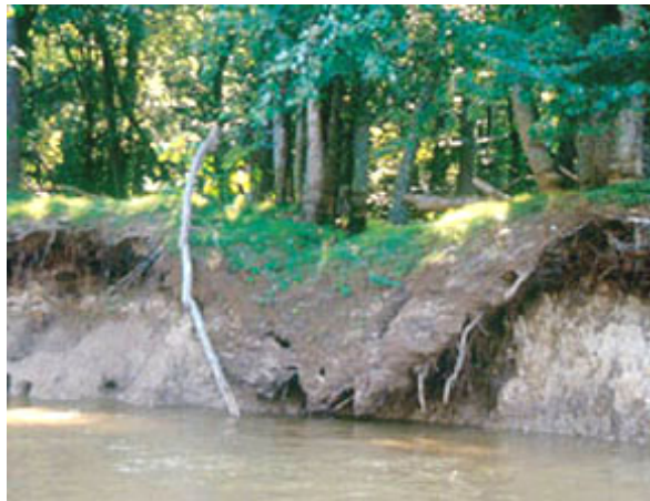
Bank Undercutting and Abrasion Thought to Result from Peaking
