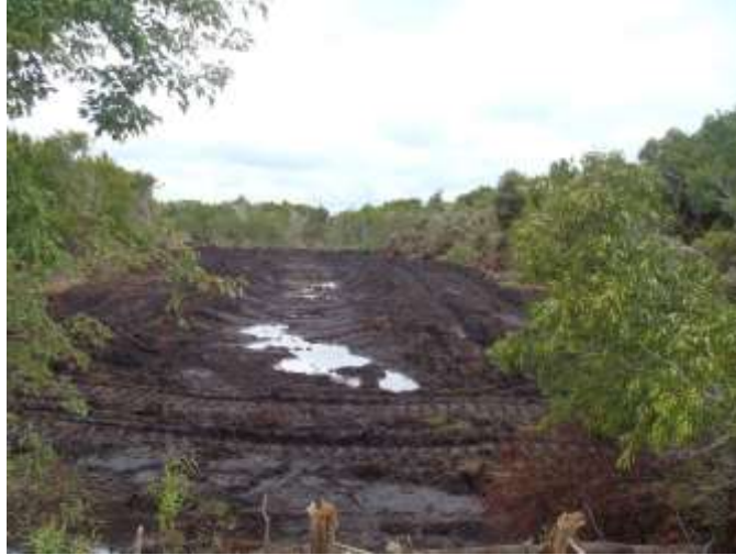
First Slough being constructed. Providing diversity of wildlife habitat and water quality benefits through increased contact with the sediments and UV exposure.
