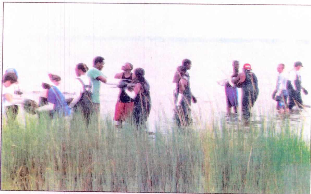
YOUTHBUILD STUDENTS traveled from Elizabeth City in May to assist with a project in Hatteras where they planted nearly 3,000 marsh grasses at a site on Durant's Point. On a second visit to the Outer Banks this month, the students helped create an off-shore sill made of oyster shell bags. This sill protects the shoreline and newly restored marsh at Jockey's Ridge State Park. (photo courtesy River City YouthBuild)
