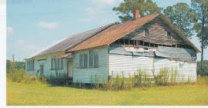
Working with the local community to preserve the historic site, the Hamilton River Partners, Inc. is working to restore and renovate the historical school. Now, the school is set for restoration for many years before the Hamilton River Partners, Inc. get involved in preparing an important part of our past.
