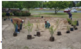
A rain garden is nature's way of cleaning up polluted runoff.
