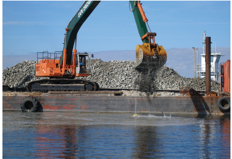
Private contractors were hired to assist in constructing over 50 acres of oyster sanctuary in 2010.
