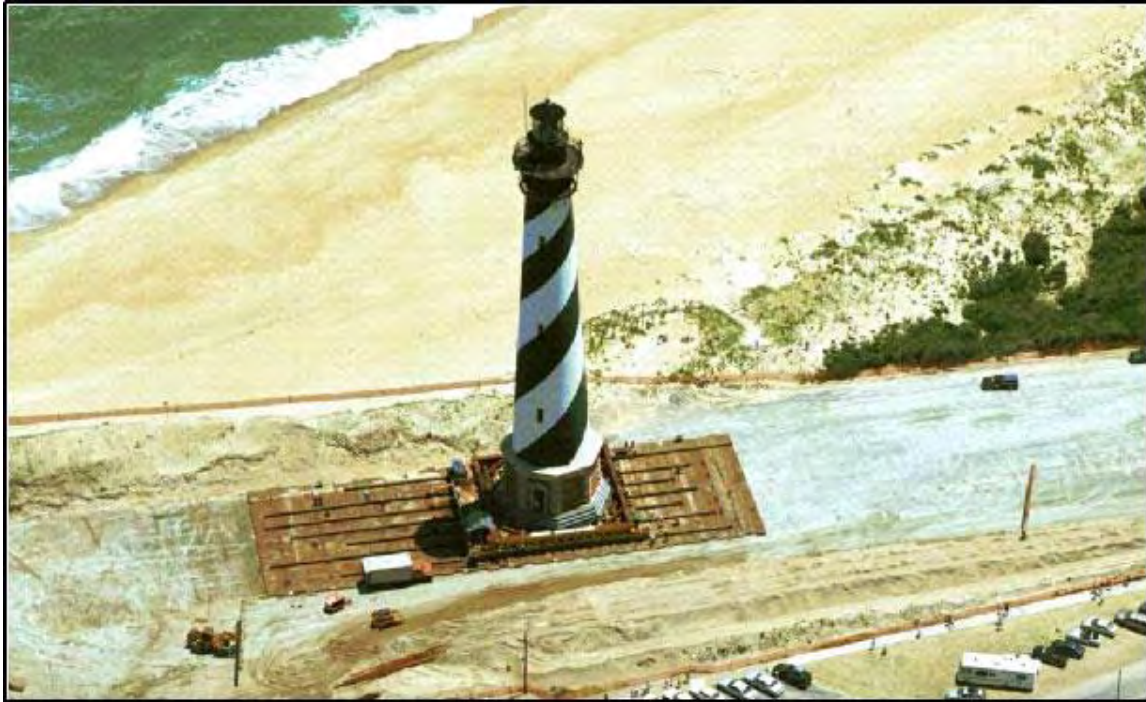
Figure 1-34. Cape Hatteras Lighthouse is on its slow and deliberate move towards the new inland relocation site. Photo is by the N.C. Department of Transportation.
