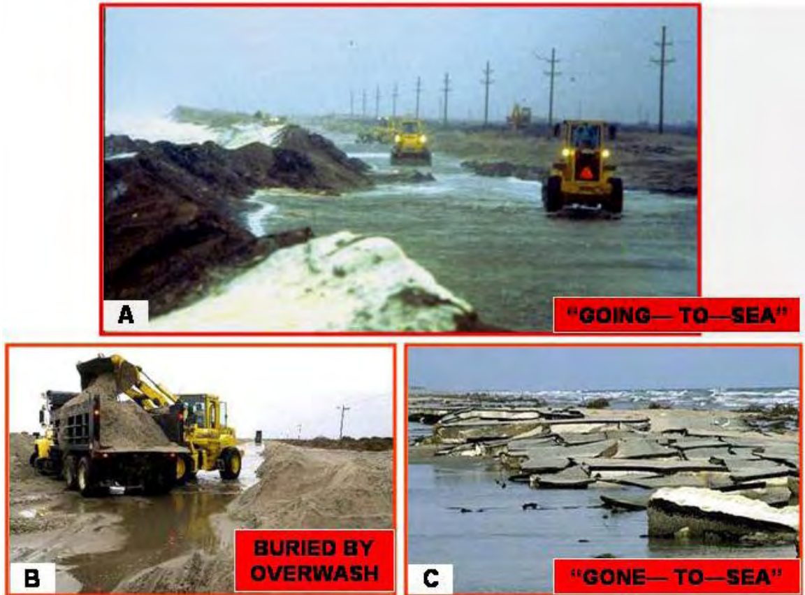
Figure 2-12. N.C. Hwy. 12 “going-to-sea” as the storm tide washes over the road during a typical nor’easter. In some storms the highway is just buried in overwash sand that is cleared off the road and put back into a barrier-dune ridge. Other storms physically destroy the road as it finds itself in the surf zone. Photograph A is by O.H. Pilkey, B is by S. Riggs, and C is by Cape Hatteras National Seashore personnel.
