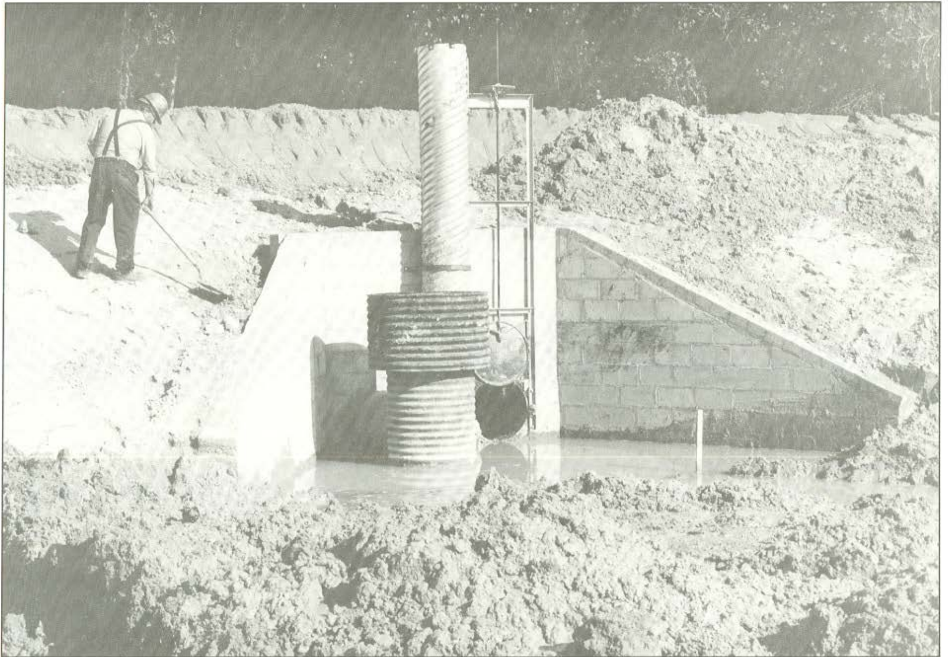
D.13. 30" perforated riser shown in center foreground. To the right of riser is handwheel-operated sluiceway.
