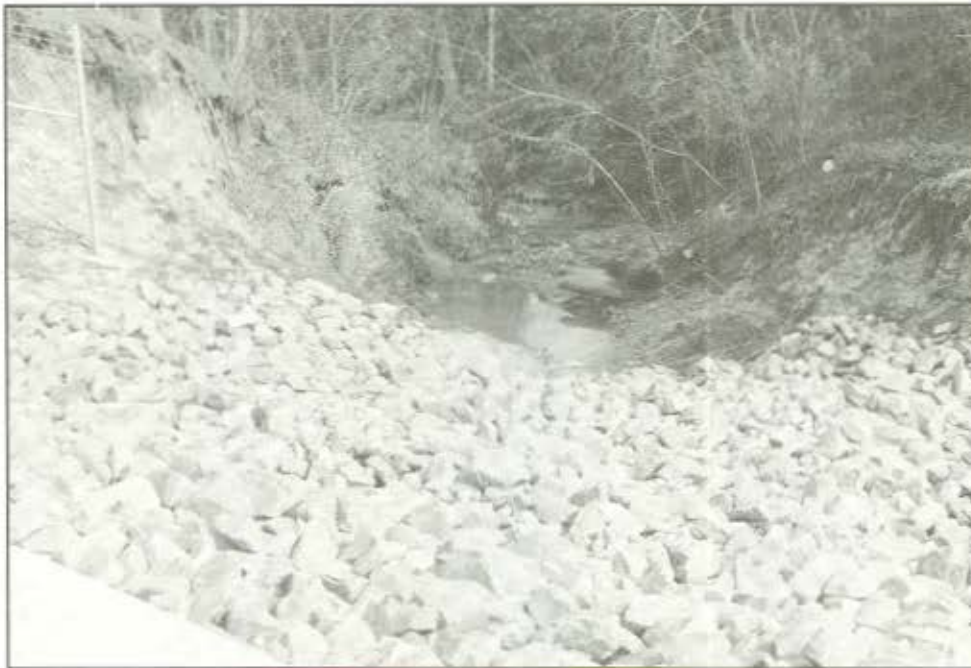
D.19. Riprap on east side of detention basin, next to spillway. Existing drainageway in background.
