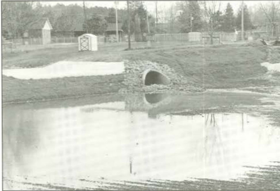
D.18. View of detention pond, facing West Third Street, showing concrete spillway, inlet discharge pipe. Storage shed contains ICMR sampling equipment.
